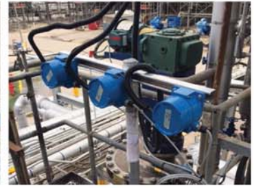
Multiple smartPIMS® Modbus DSI networked for monitoring dozens of TMLs.
