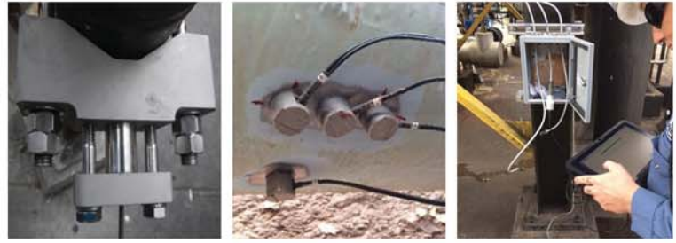
Clamped high-temp probe monitors ~640°F line. • Dual-element probes monitor individual pits. • Datalogger cable runs to enclosure for data collection.
